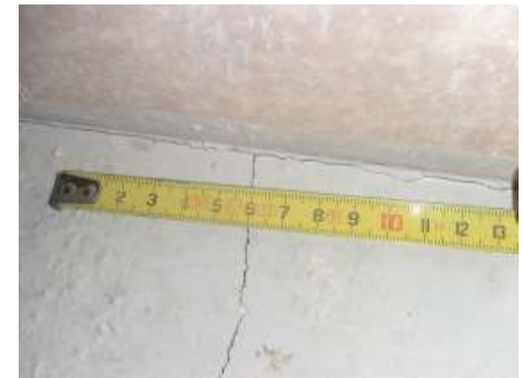
Tear at the surface with ~1mm opening
